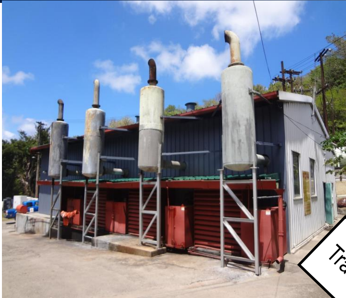
Diesel Generator Power Plant in Bequia
